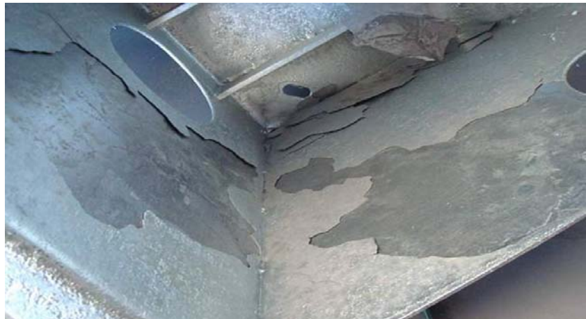
Photo 2 Poor galvanizing due to steel chemistry
