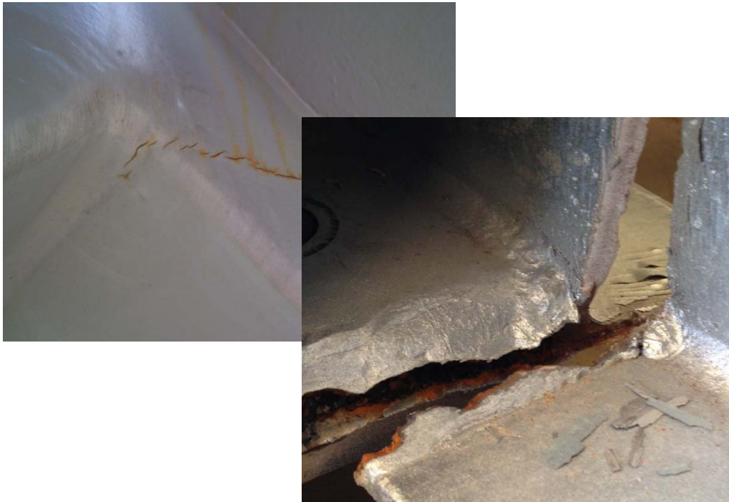
Photos 7–8 Steel cracking on imported fabricated product
