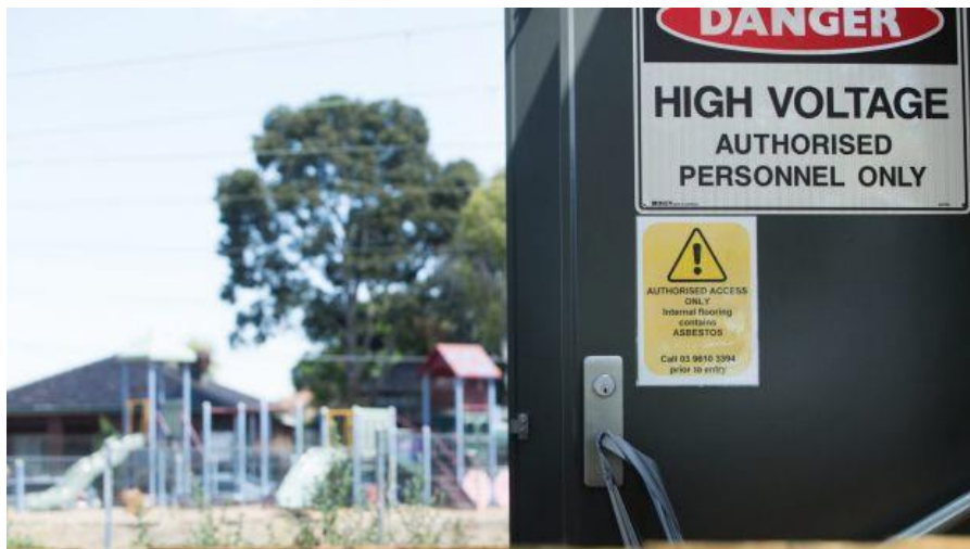
The Thornbury substation, with the childrens' playground in the background. Photo: Simon Schluter
