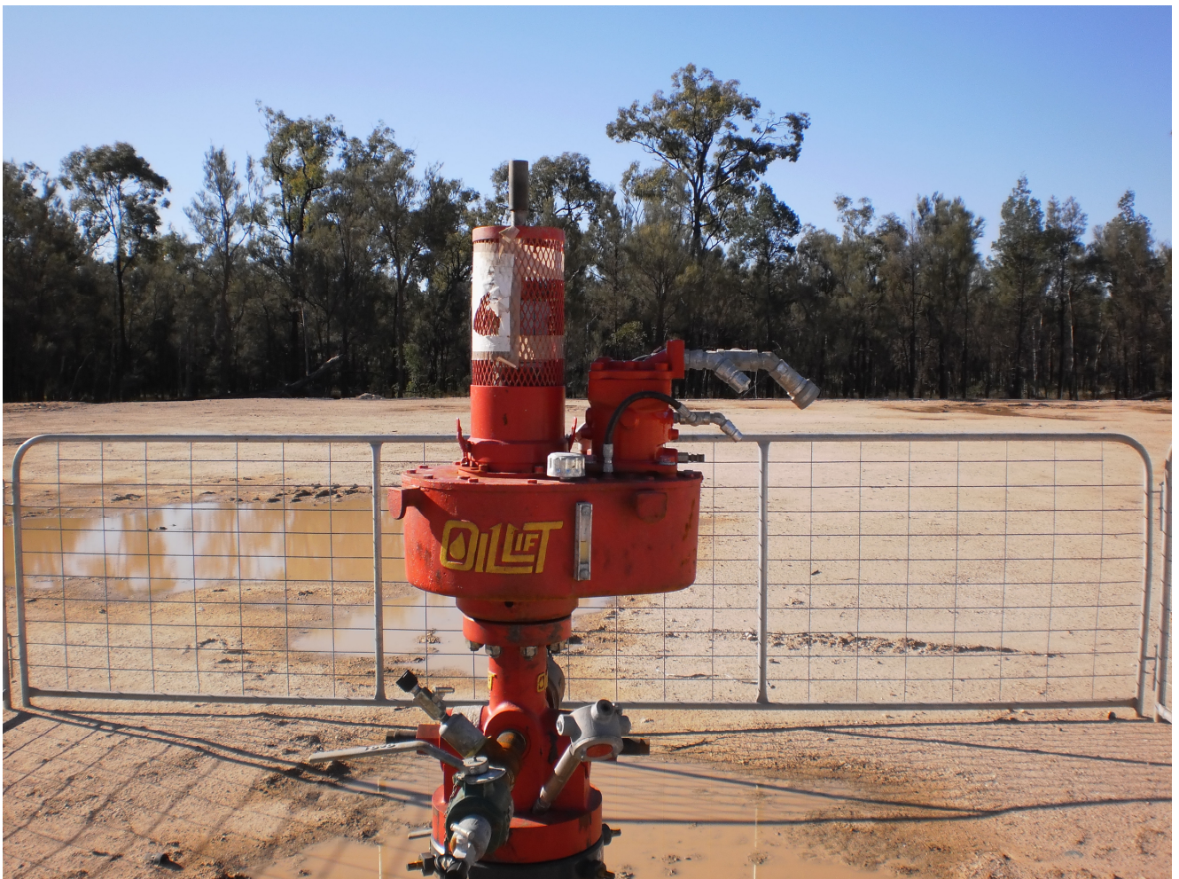
A gas well in Condamine State Forest with a 100m x 100m clearing around it
