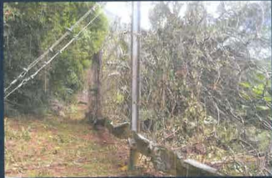
Seven rockfall fences and five berms protect the Kampong at Flying Fish Cove.
