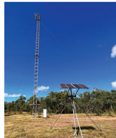
HCRC microwave tower in Gängaṅ homeland
