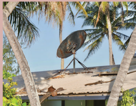
Rusted VAST satellite dish on house in Erub
