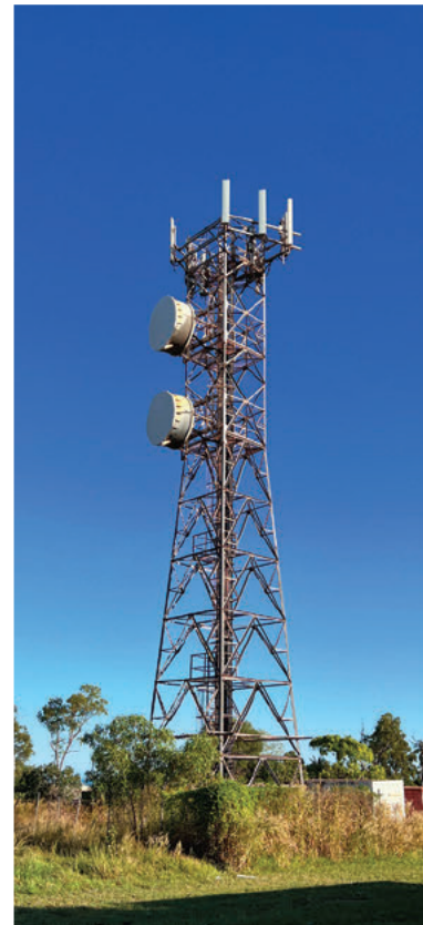
Mobile tower at Galiwin'ku
