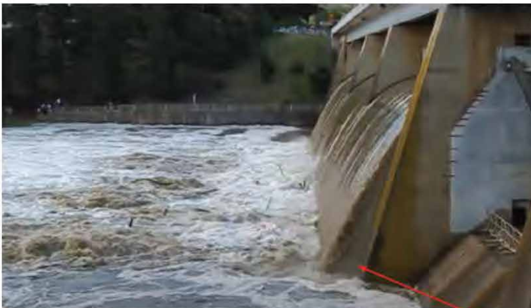
Figure 12 Water surface profile relative to the shape of the piers and end training walls
