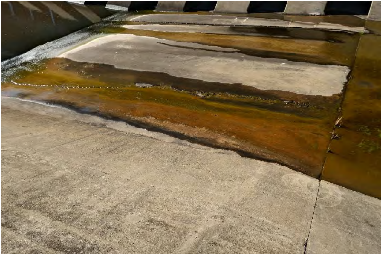
Photo B- 2.23 – Typical cracking Bay 4
