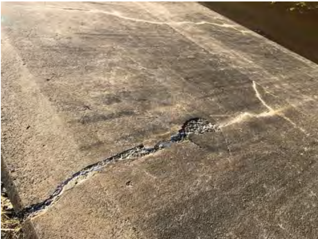
Photo B- 2.26 – End sill Cracking
