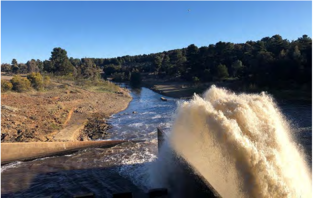
Photo B- 3.3 – Sluice in Operation
