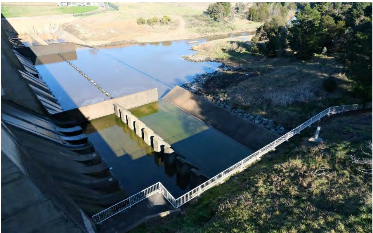
Photo B- 2.18 – Downstream view of top of right training wall looking towards stilling basin
