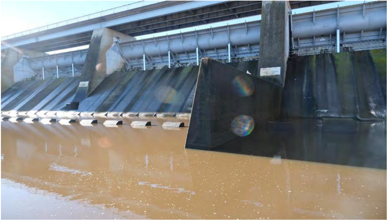
Photo B- 2.11 – Stilling Basin divider/ splitter wall
