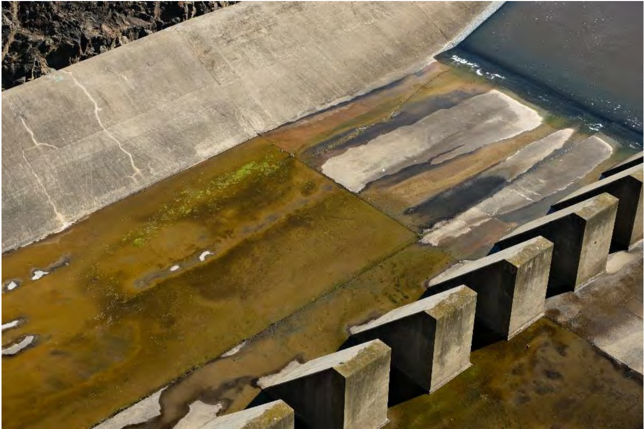
Photo B- 2.25 – Typical Crack Bay 4 and 5
