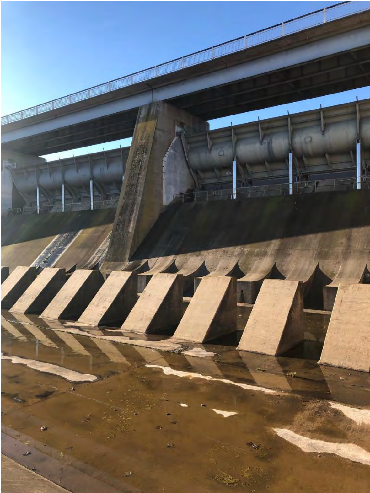
Photo B- 2.27 – View of Chute blocks, apron and baffle piers and Spillway Gate
