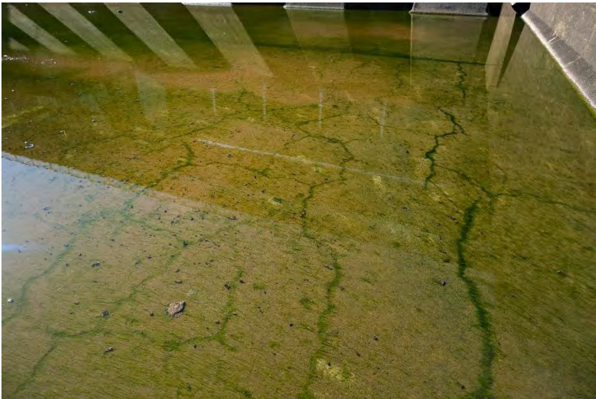
Photo B- 2.24 – Typical Cracking Bay 1
