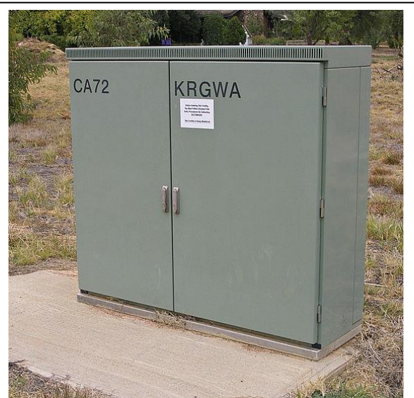
Figure 1: Example of a roadside cabinet
