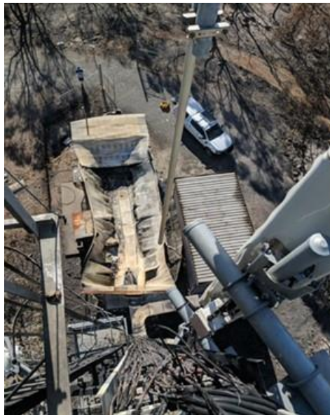
Figure 2: Fire-damaged mobile network facility, Mount Torrens SA
