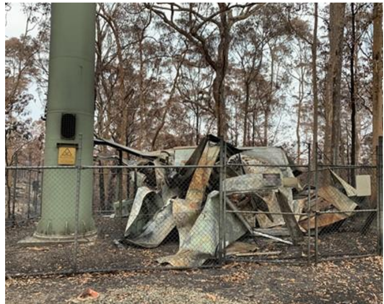
Figure 3: Fire-damaged mobile network facility, Surf Beach NSW
