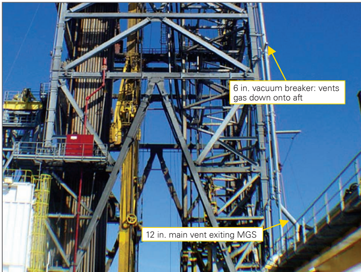
Figure 5. Photograph of 6 in. Vacuum Breaker Line Gooseneck Vent.
