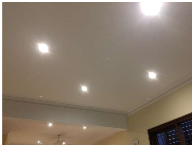
Figure 13 - Efficient LED lighting throughout
