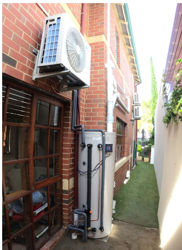
Figure 9 - Air Source Heat Pump for hot water
