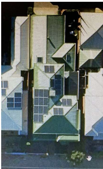
Figure 4 - Solar PV - 1.5kW facing East, 1.8kW facing North, 3.3kW facing West
