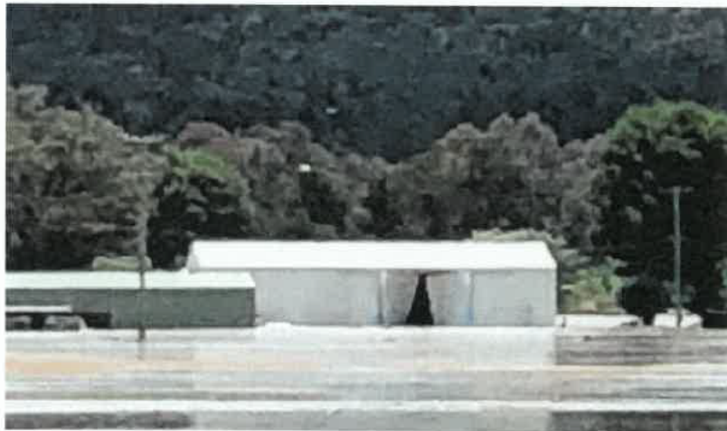
Photo 8: Image of a machinery shed on the subject property. The photo shows the eastern facing side of the shed and a set of double doors that have been pushed inwards. Had the water only originated from the north, those double doors would not have been pushed inwards, rather outwards due to excessive water entry into the shed from the north (source: personal image taken of subject property from Hillview Ln).
