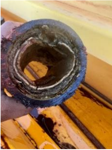
1. Sewer pipe showing build up
