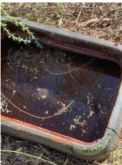
3. Potable water pit with leak
