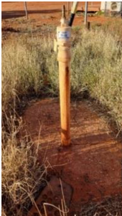
2. Fire hydrant missing connector
