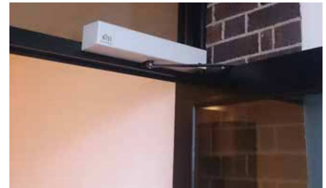
Automated apartment doors, showing internal wall button for automatic door opening (above), and typical door automation hardware (below), Abbotsford.
