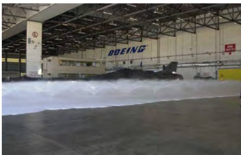
Figure 2.2. Activated AFFF foam sprinkler system test forming a foam blanket on the hangar floor.
