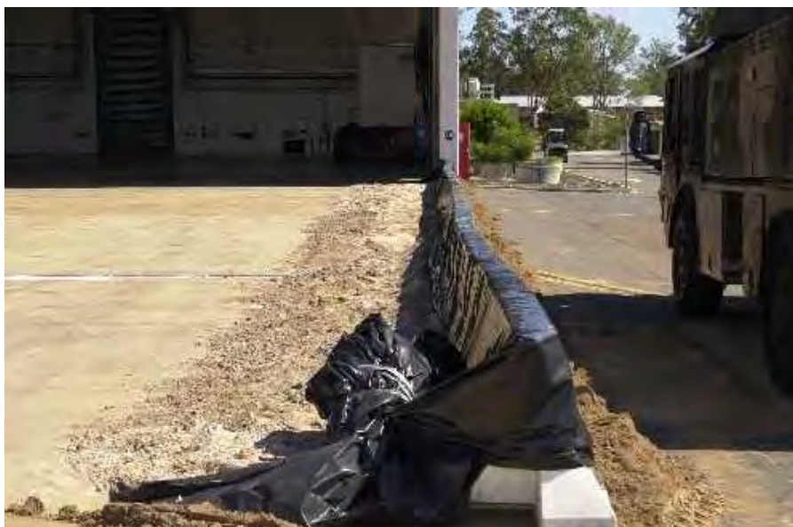
Figure 4.4. Temporary bunding outside a RAAF Amberley hanger in preparation of foam discharge during the testing of a hangars AFFF system.
