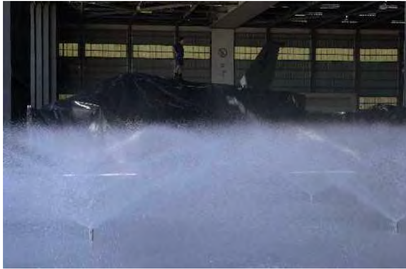
Figure 4.2. An activated pop-up sprinkler foam system
