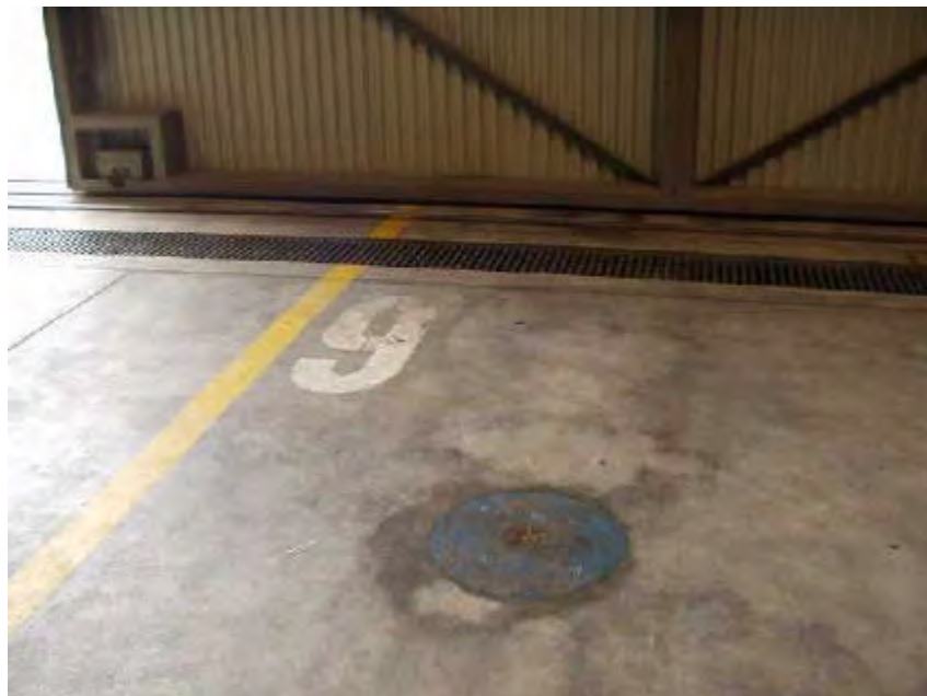
Figure 4.3. AFFF waste-water drainage grates located inside the hangar
