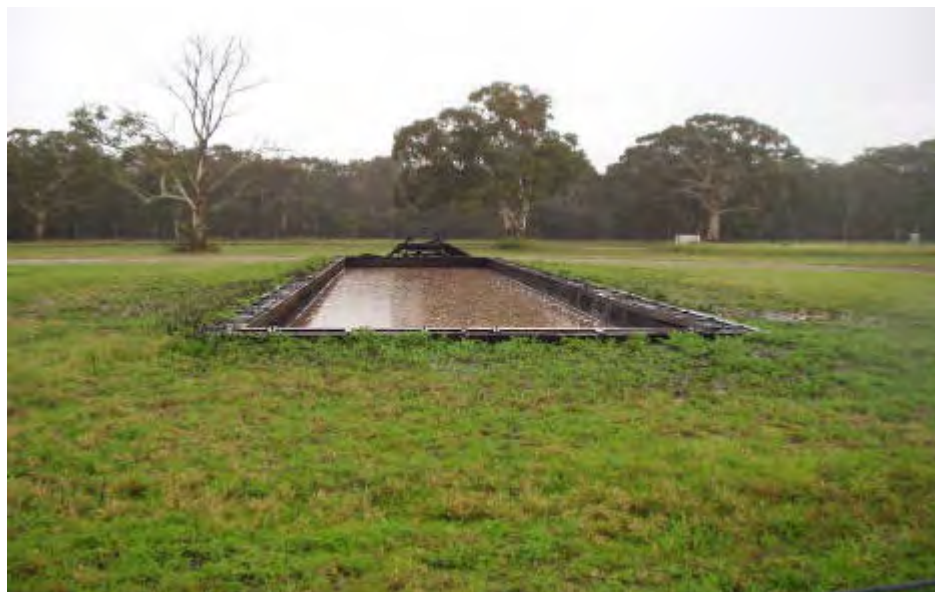
Figure 4.8. An example of a hot fire training pit at RAAF Williamtown. This pit does not have any controls to prevent spillage of fuel or AFFF flowing onto surrounding soil/grass areas.
