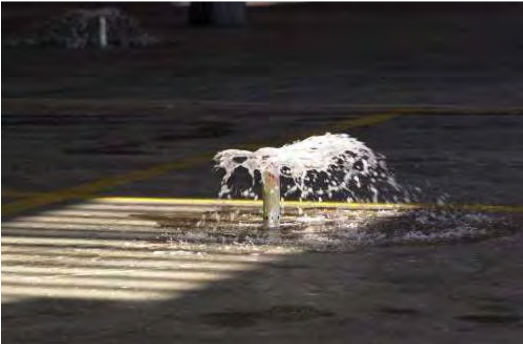
Figure 4.1. A pop-up sprinkler on the floor of a hangar, a few seconds after the foam system was activated.
