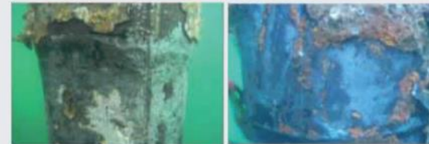
Steel pile corrosion and exposure of concrete
