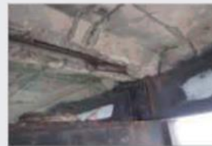
De-lamination of concrete and corrosion to steelwork
