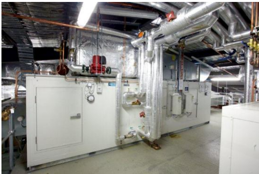
1. Specialised air handling systems ensure sterile air is passed into the compounding facility
