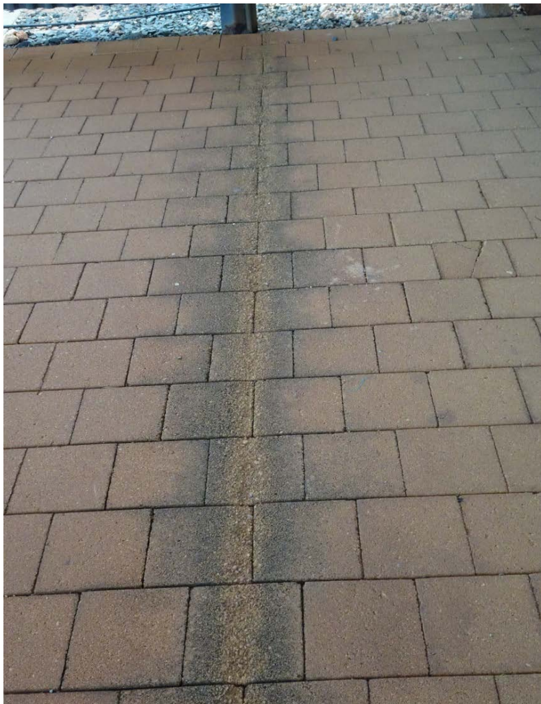
Figure 2: Effect on brickwork of 'acid rain' from gap in roofing at Woodside Visitor Centre, July 2016
