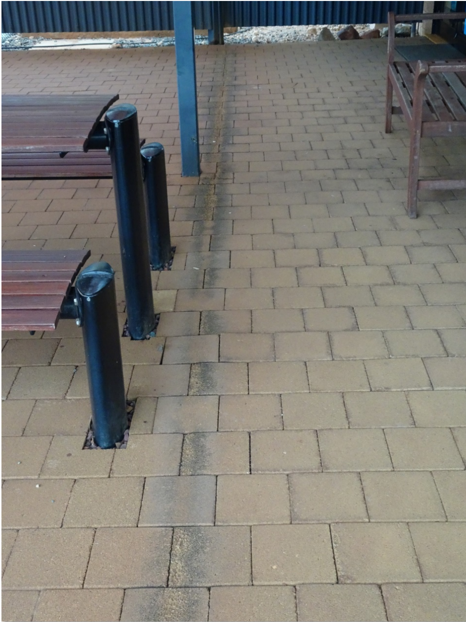
Figure 3: Effect on brickwork of 'acid rain' from gap in roofing at Woodside Visitor Centre, July 2016
