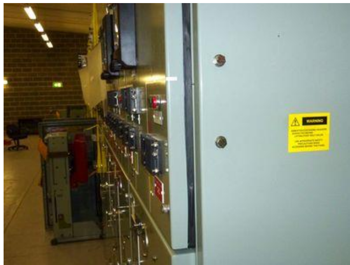
Electrical switchgear equipment inside an Ausgrid substation
