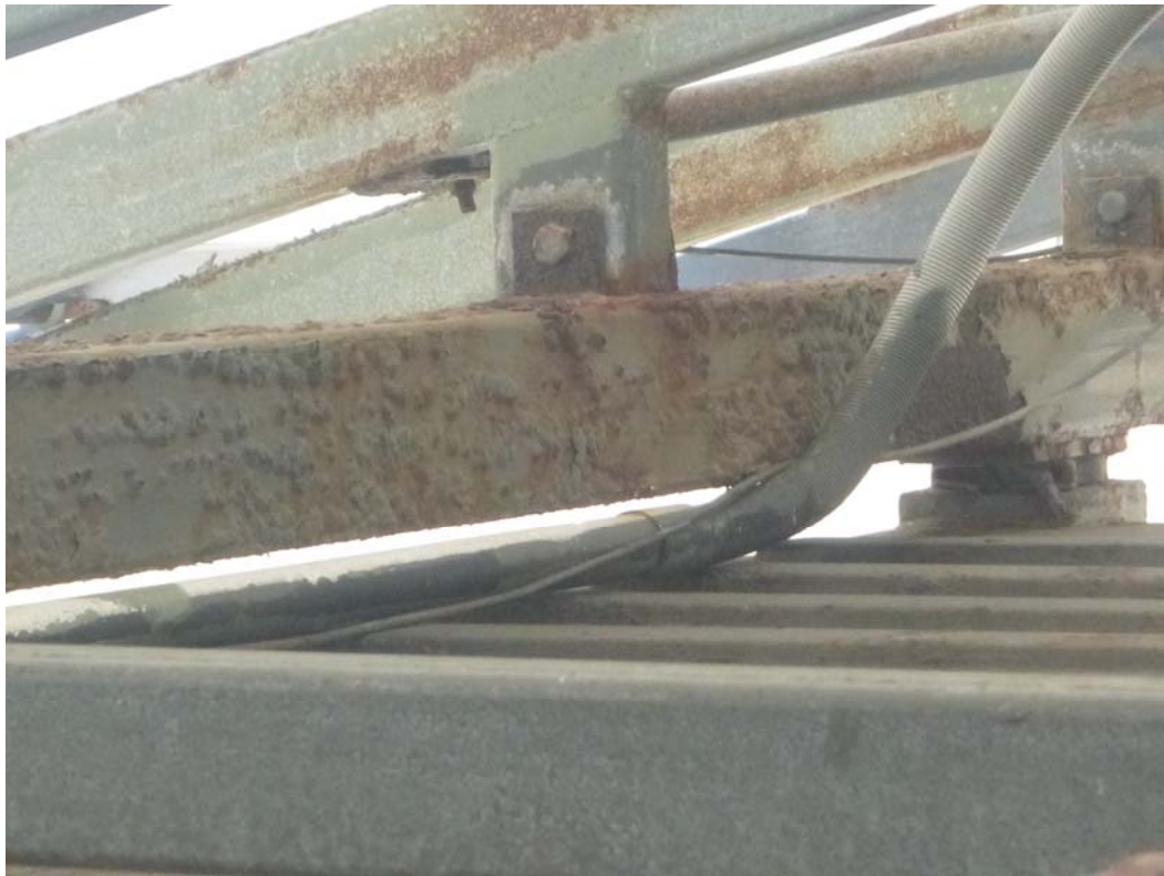
Figure 3: Examples of corrosion issues and damage at the existing temporary ARFF facility at Hamilton Island
