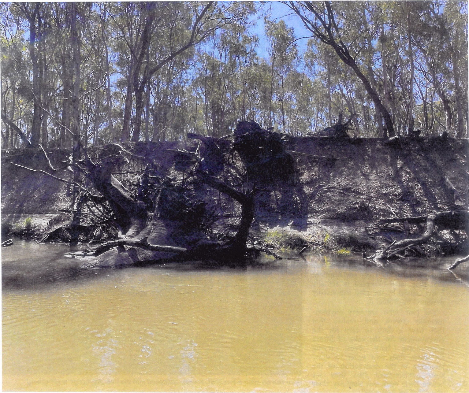
In this photo the erosion of the bank of the Edward River can be clearly seen. This erosion results in large trees having their roots undercut, causing them to collapse into the river where they end up clogging up the waterway.
