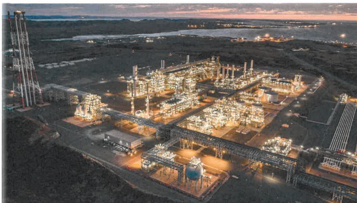
Woodside is expanding its Pluto LNG plant in Western Australia through gas from its offshore Scarborough field. Picture: Woodside
