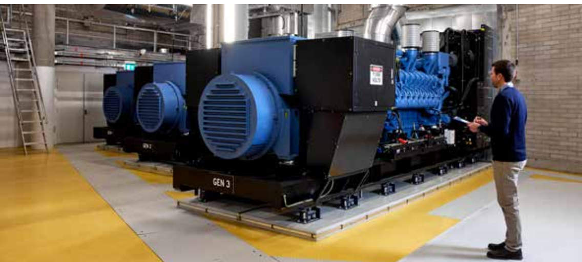
DPS staff member records test data from one of the new auxiliary generators. Photo credit: Lightbulb Studio.
