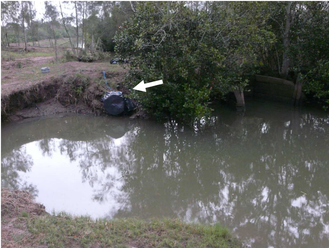
Figure 3. Reinforced plastic was placed over the overflow pipe (arrow) to prevent water escape.
