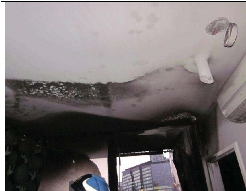
View of damaged wall and smoke detectors made inoperable. Others were covered over.
