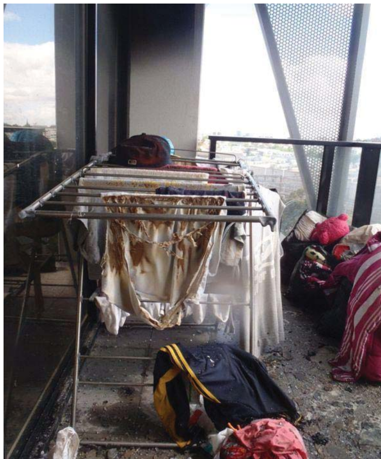
Figure 11 - Combustibles stored on one of the balconies.
