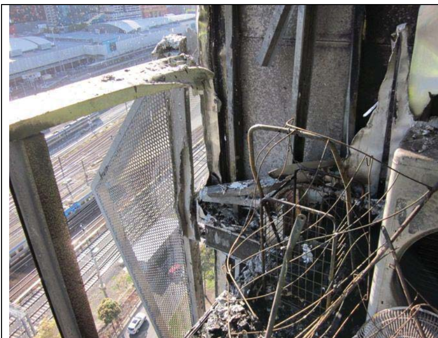
Wall between bedroom and balcony. Construction lightweight wall with steel studs, aluminium type external cladding plasterboard to internal. Material stored on balcony.
