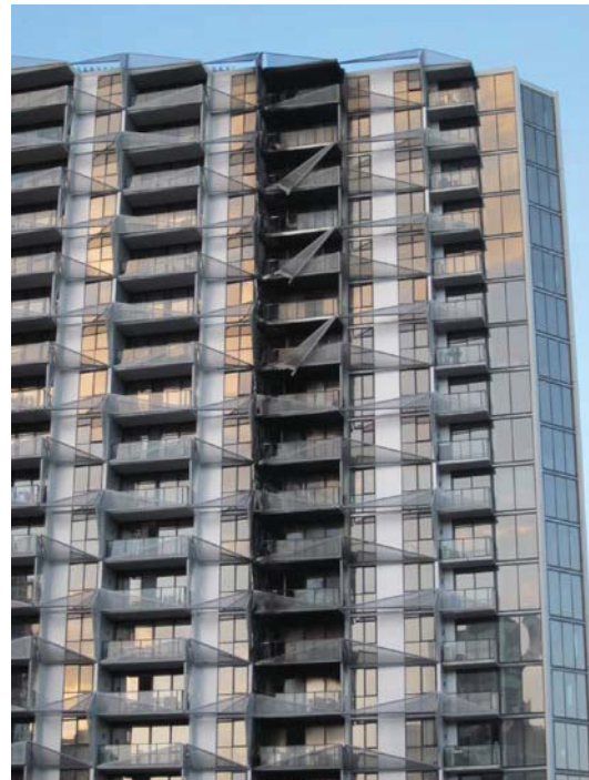
Photo Post Fire
