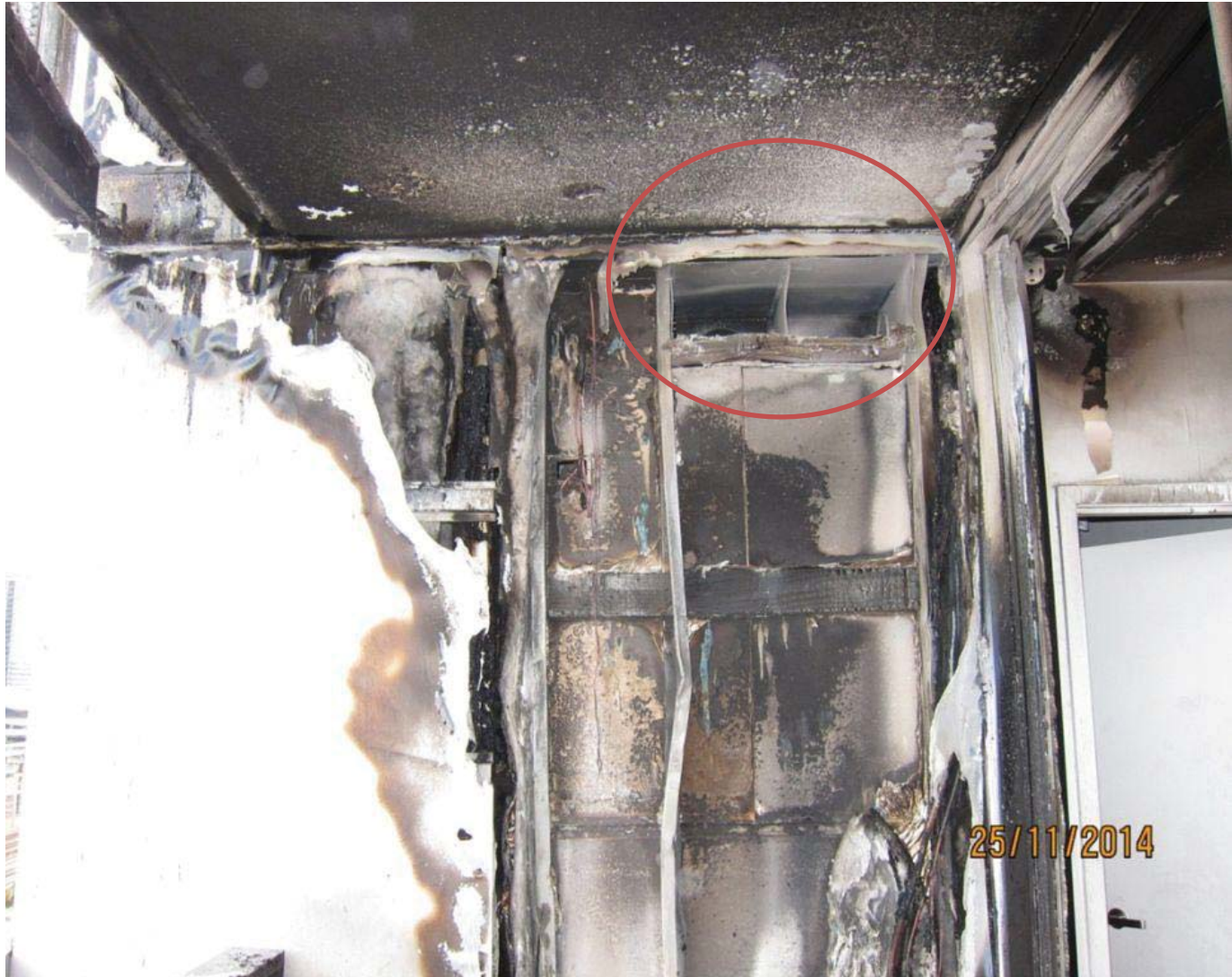
Figure 19 - Apartment Exhaust Duct
