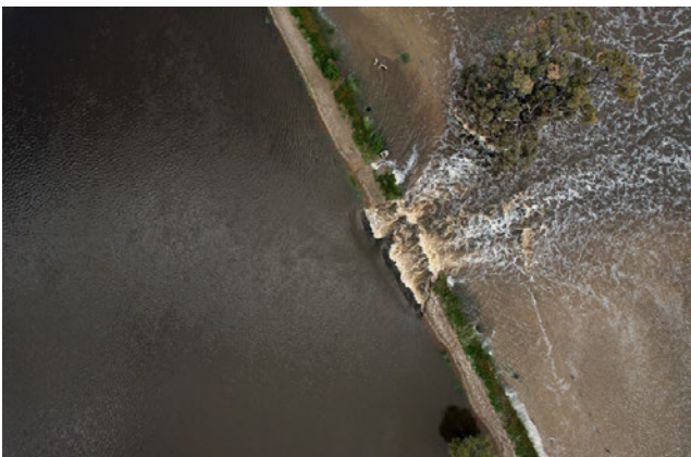
Burst levee bank. Photo taken by Jason Saraj.
