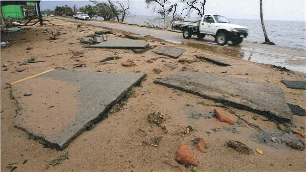
Road damage from Cyclone Yasi in Cardwell, far north Queensland, in 2011. RICK RYCROFT/AP
